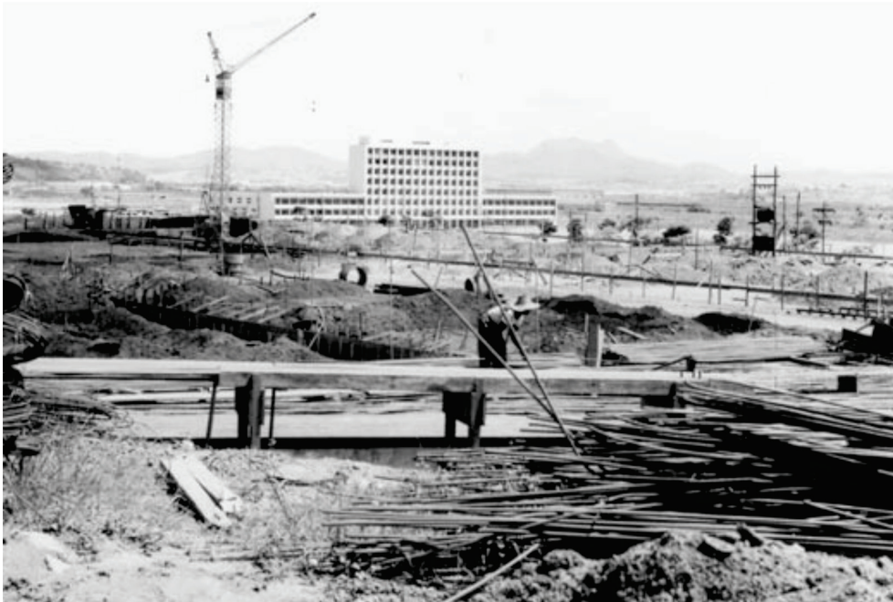
FIGURE 2 – Geography and History building under construction, in 1964. Author: unknown. Source: CCS, Jornal da USP .
